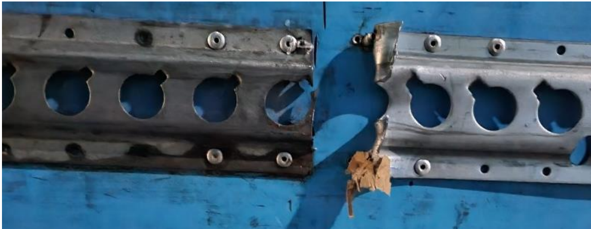
Figure 4: Damaged load restraint in a refrigerated vehicle
